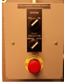
212A Emergency Power Kill Switch
